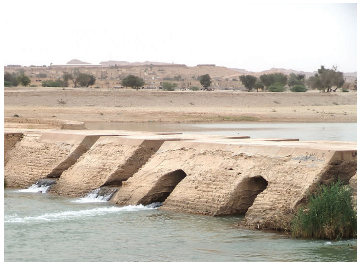
Pic 2: Mizan Dam: this dam divides the Karun water by ratios of 2:1 between Gorgor and Shatit rivers respectively. Gorgor River is called Dodangeh or Masroqan (the handmade river) as well as Shatit River is called Chohardangeh. This dam is in such a way that, if the water discharge of Gorgor is more than one third, transfers the excess water to Shatit branch. Source: www.fa.wikipedia.org .
